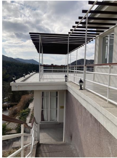
Figure 9 – Photograph showing the wooden beam additions on the terrace area. The photograph was taken from the stairs that lead to the upper floor of the building. The landing of the staircase serves as the entrance platform. (Photograph taken by the author)
