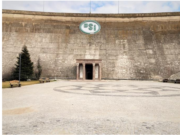
Figure 4 – Photograph showing the current view of the portico as attached to the curved structure of the dam with its classical architectural elements.
